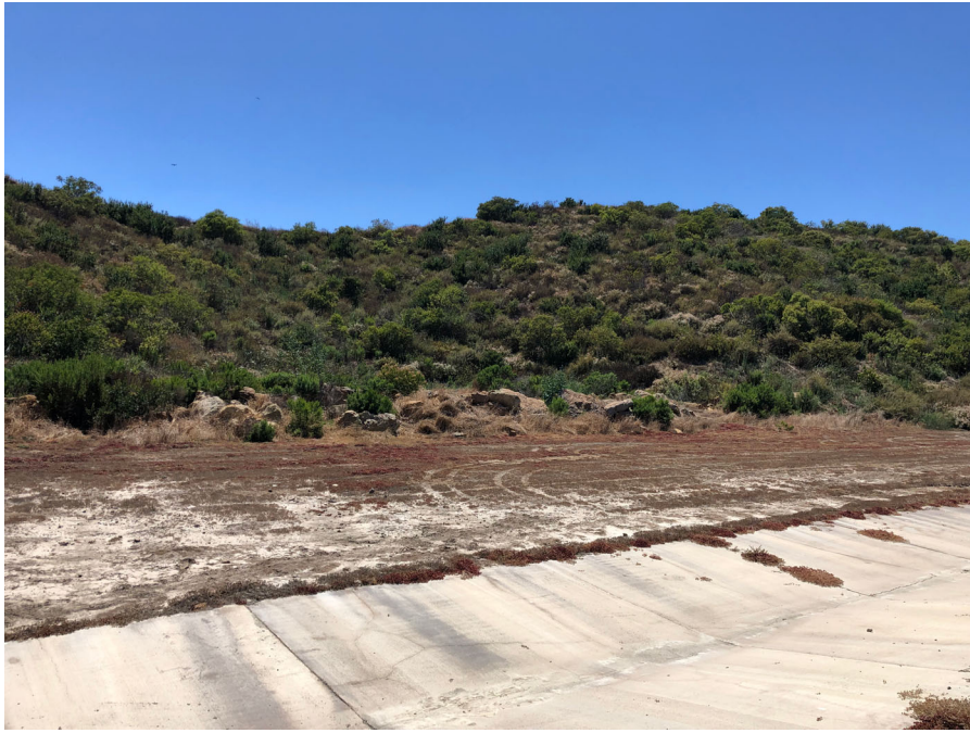
View of the concrete v-ditch and coastal sage scrub restoration area located to the west of the project site. July 16, 2019.
